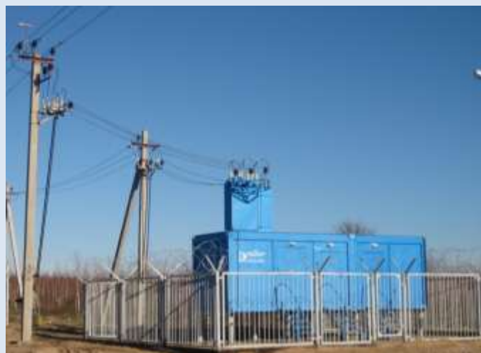
Block container power plant
