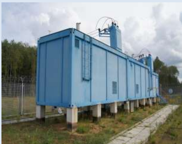
Micro turbine unit
