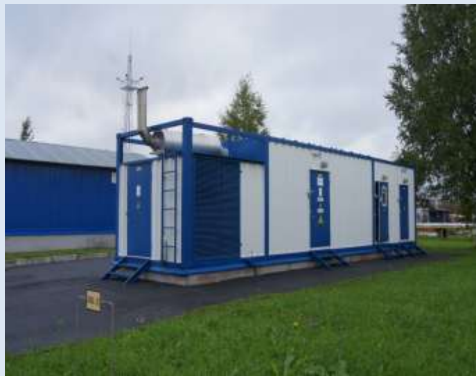
Autonomous diesel-engine power plant
