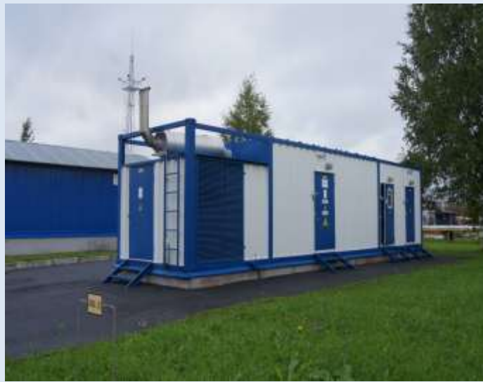
Autonomous diesel-engine power plant
